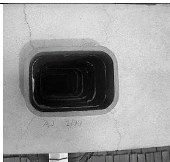
Clay Tile Liner Flue
