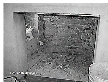
Badly Deteriorated Firebox
